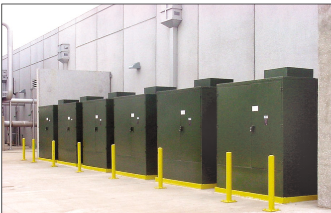
Main feeder transformers keep ISP on-line 24/7.
